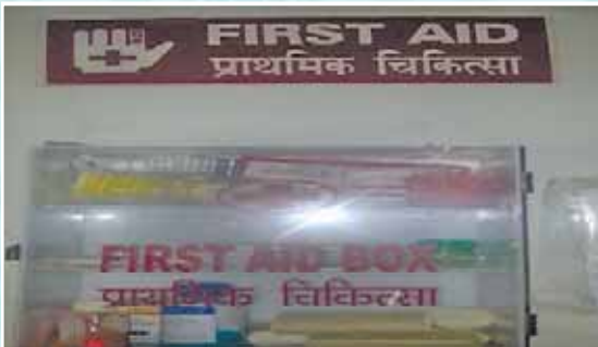
Fully Equipped First-Aid Box at Shop Floor
